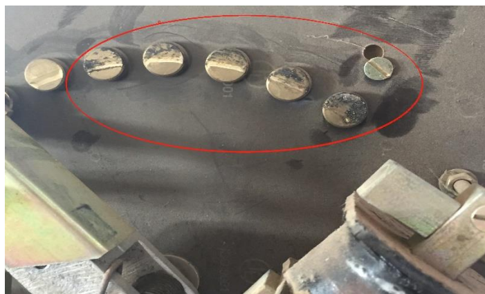
Figure 7: Sparking in conventional starters
