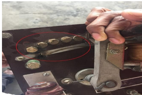
Figure 6: Corrosion of conventional starters
